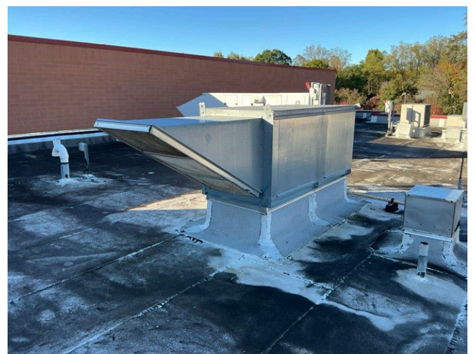
30 - MAKE-UP AIR UNIT
