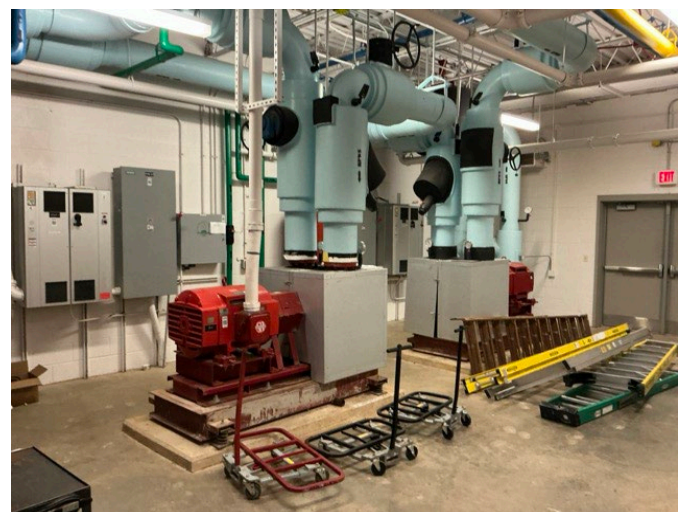
24 - MAIN MECHANICAL ROOM
