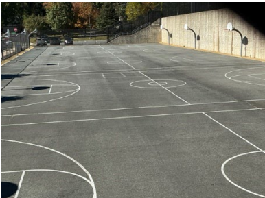
Backboard missing - AssetCALC ID: 9956914
