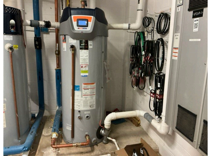
26 - CONDENSING GAS WATER HEATER
