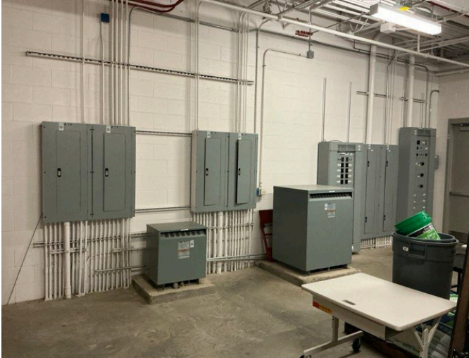
25 - MAIN ELECTRICAL ROOM
