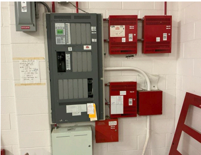
33 - FIRE ALARM PANEL
